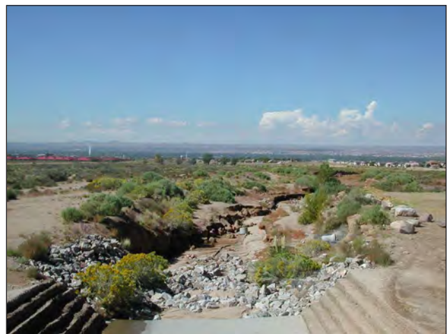
Window G Channel releasing into Park site
